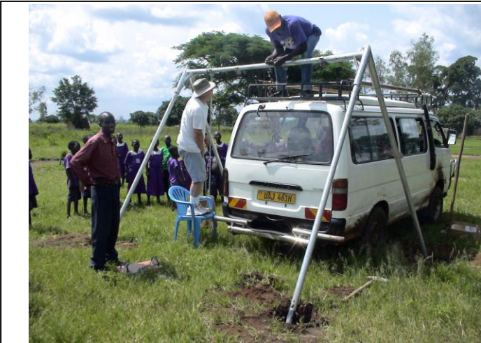
Roger and Kent have a long-term program to install recreation equipment at orphanages and schools. This is the beginning of an installation at Aromo. They designed end brackets that can be fabricated locally, and as you can see, innovative methods are used for installation in the field.
