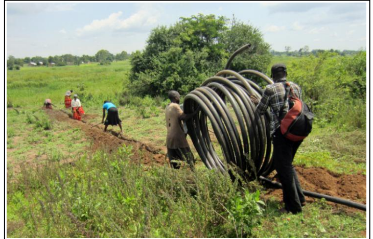
One hundred meters of 2-inch HDPE pipe was installed after women dug the trench. One inch diameter laterals were added to deliver water to hose spigots and movable sprinklers.
